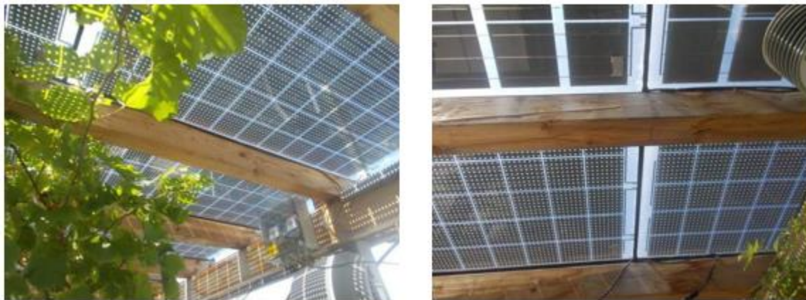
Figure 6. Rooftop with Photovoltaic Panels at the University für Bökdenkultur, Vienna, Austria 2016
